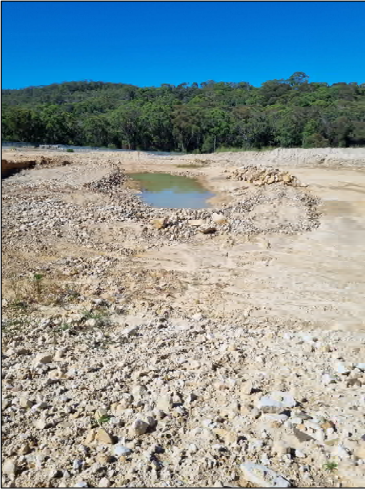
Photo C.5 View of the sediment pond in the south west of the project site (facing south)
