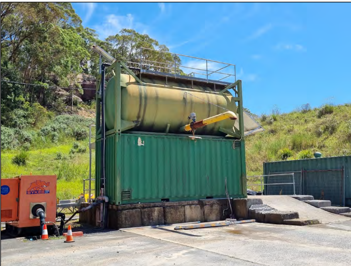
Photo C.8 View of the 'structures' on the project site – AST and storage tanks
