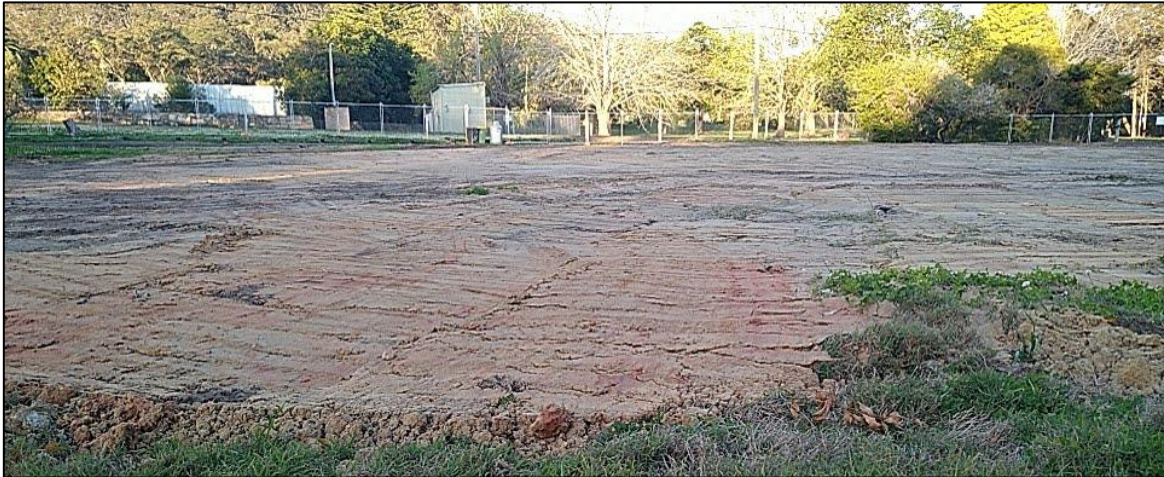
Figure 7: Fill observed in the locality of the former structures. Photo taken 6 September 2021.
