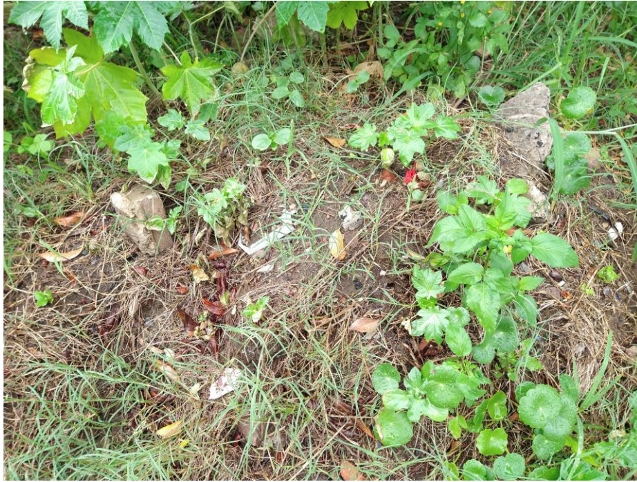
Photo 7 – Mounded area with building rubble on the surface
