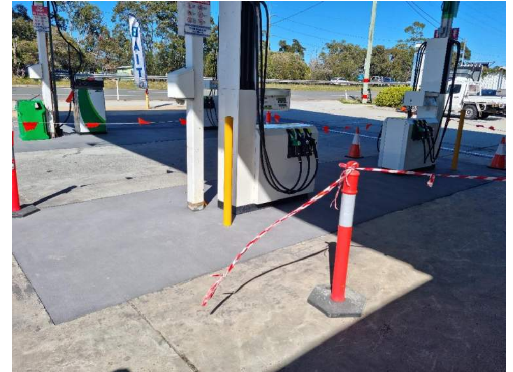
Photo 27: Two bowsers currently not in operation, with newly laid concrete at their bases.
