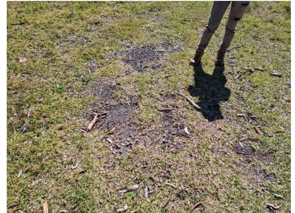
Photo 12: Asphalt patch (approximately 3m x 3m) located on the northern end of Lot 83, suggesting a previously built structure has since been removed.
