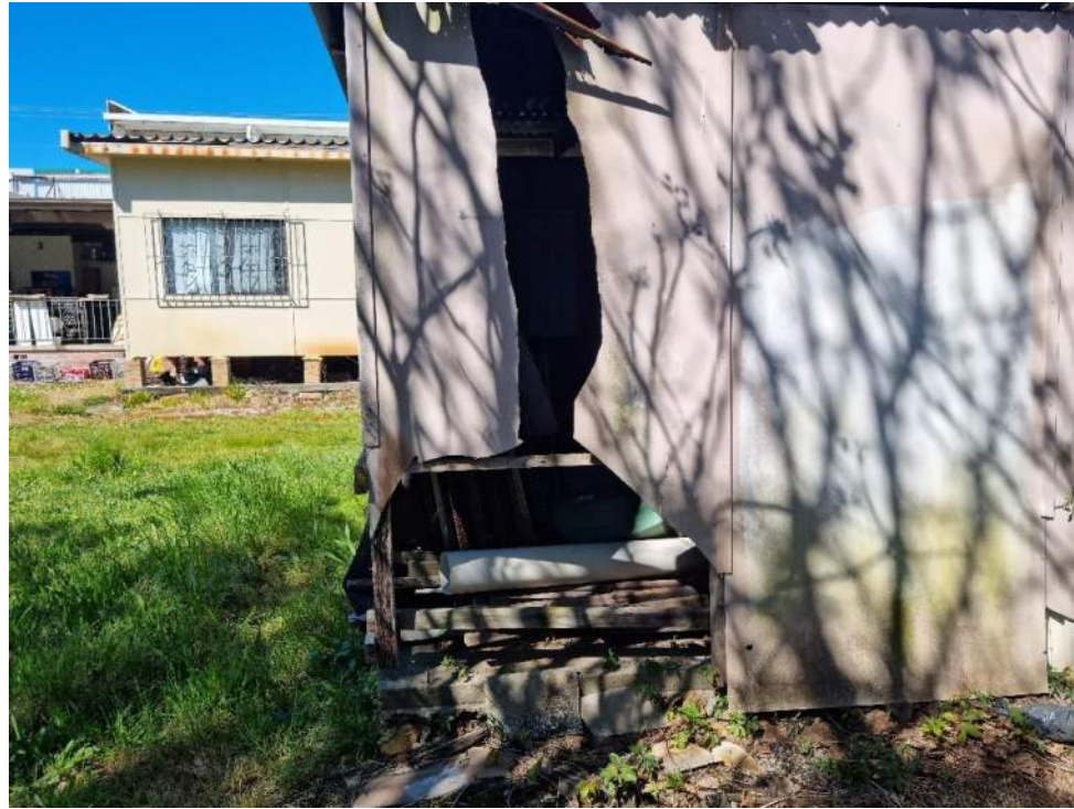
Photo 37: A second shed at the back of the main site buildings that appears to be in poor condition with broken walls exposing the contents.
