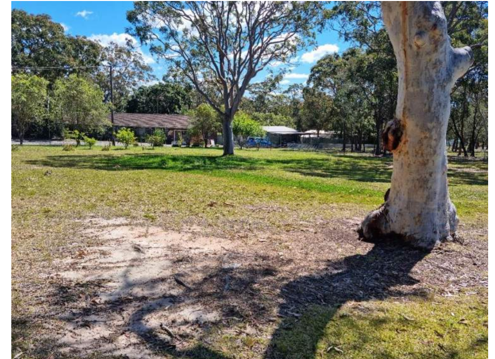
Photo 9: Exceptionally green grass trailing west from the septic tank, indicating a potential leak.
