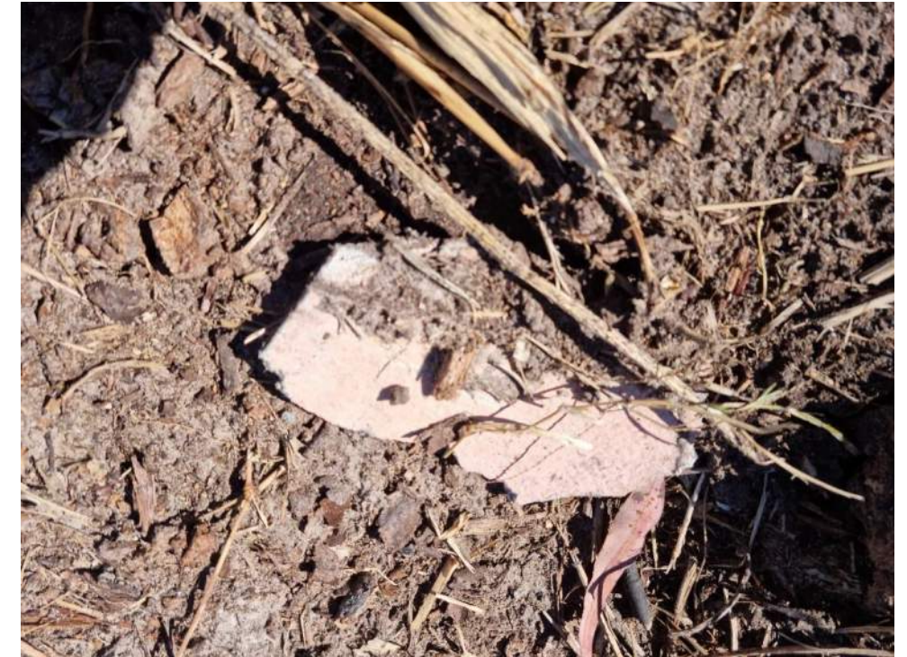
Photo 15: Potential ACM found amongst the fill material in the soil stockpile from Photo 14.
