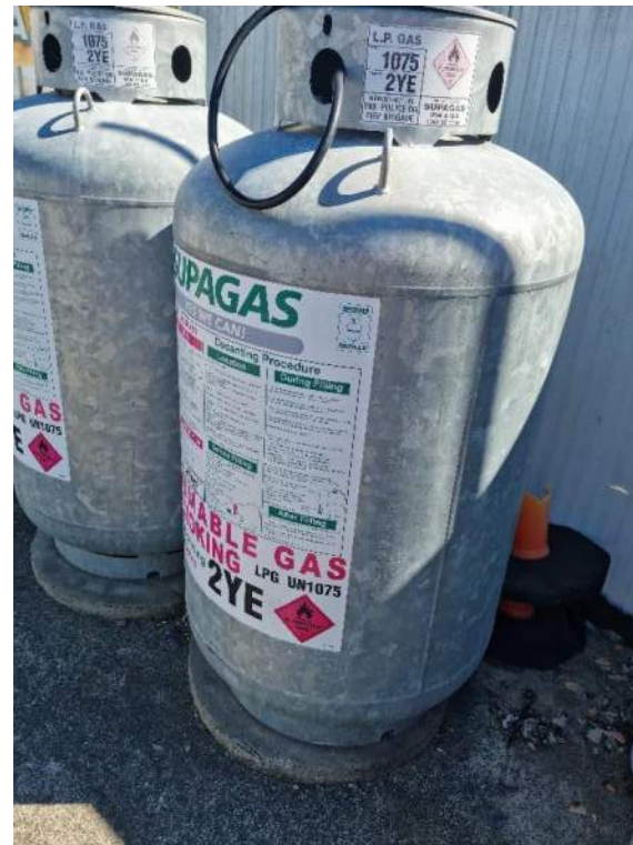
Photo 29: Two large LPG gas tanks located in the north-west corner of Lot 12
