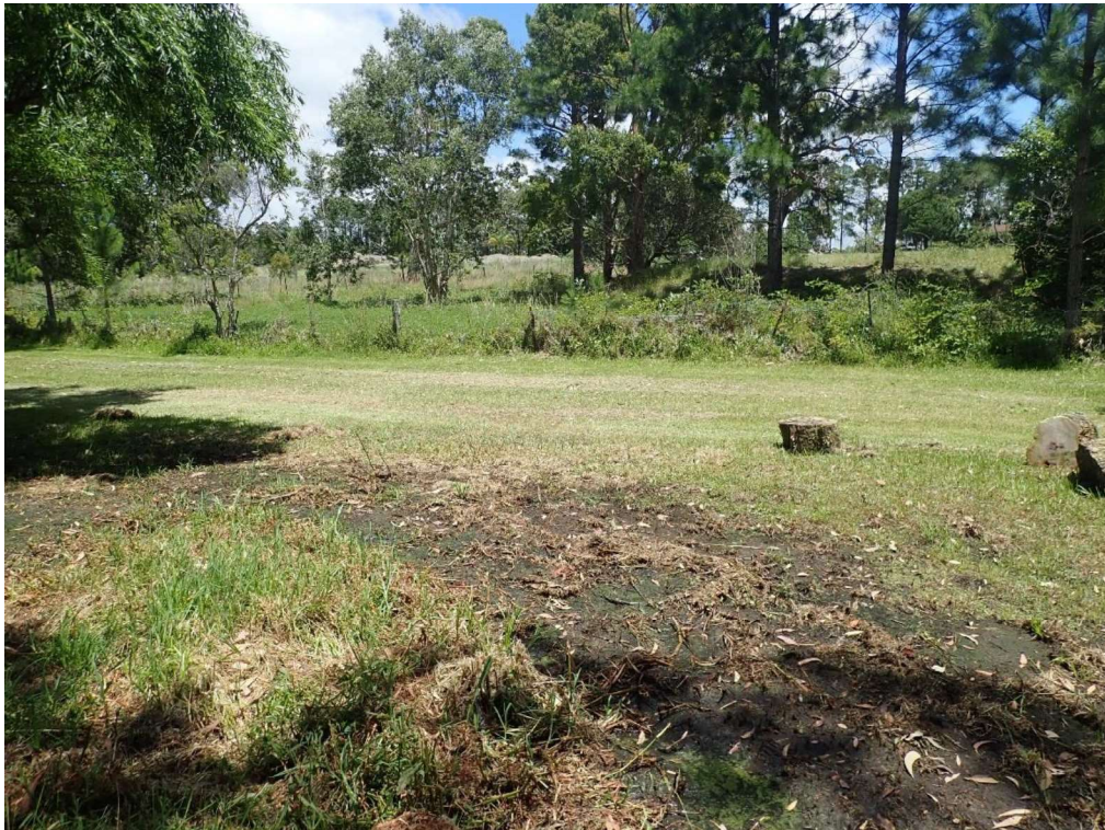
Photo 16 – Saturated ground (seepage point) on No. 305 east of Dam 2 (northern dam) located on No. 295
