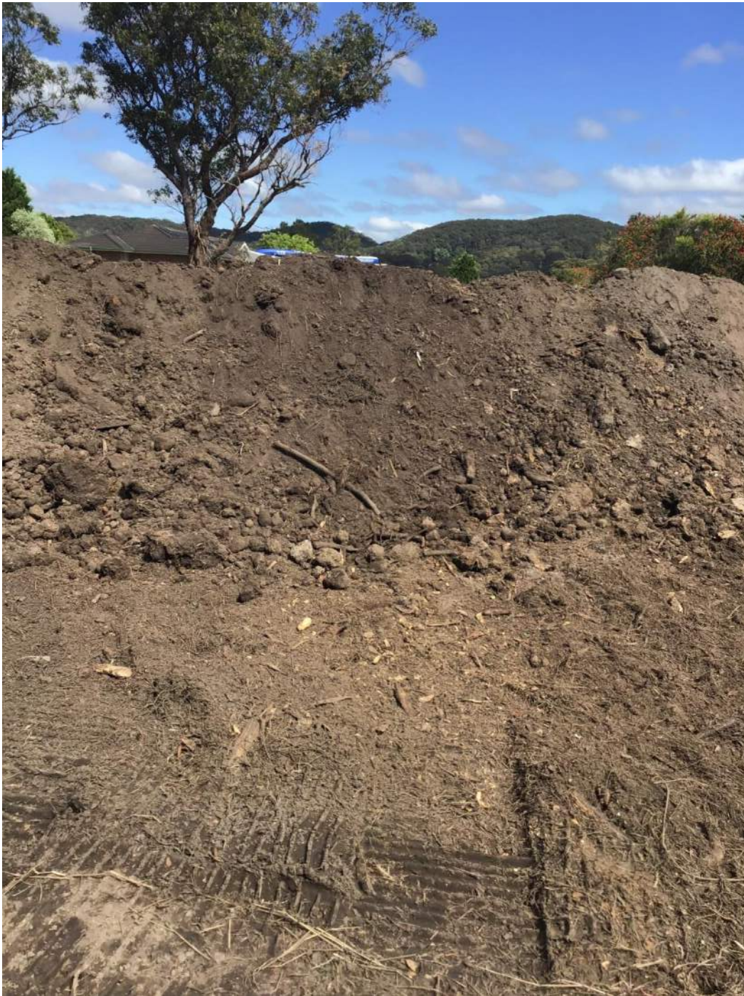
Photograph 8: Recent Stockpile Dumping (see OIN 10 on Figure 2 in Appendix A).
