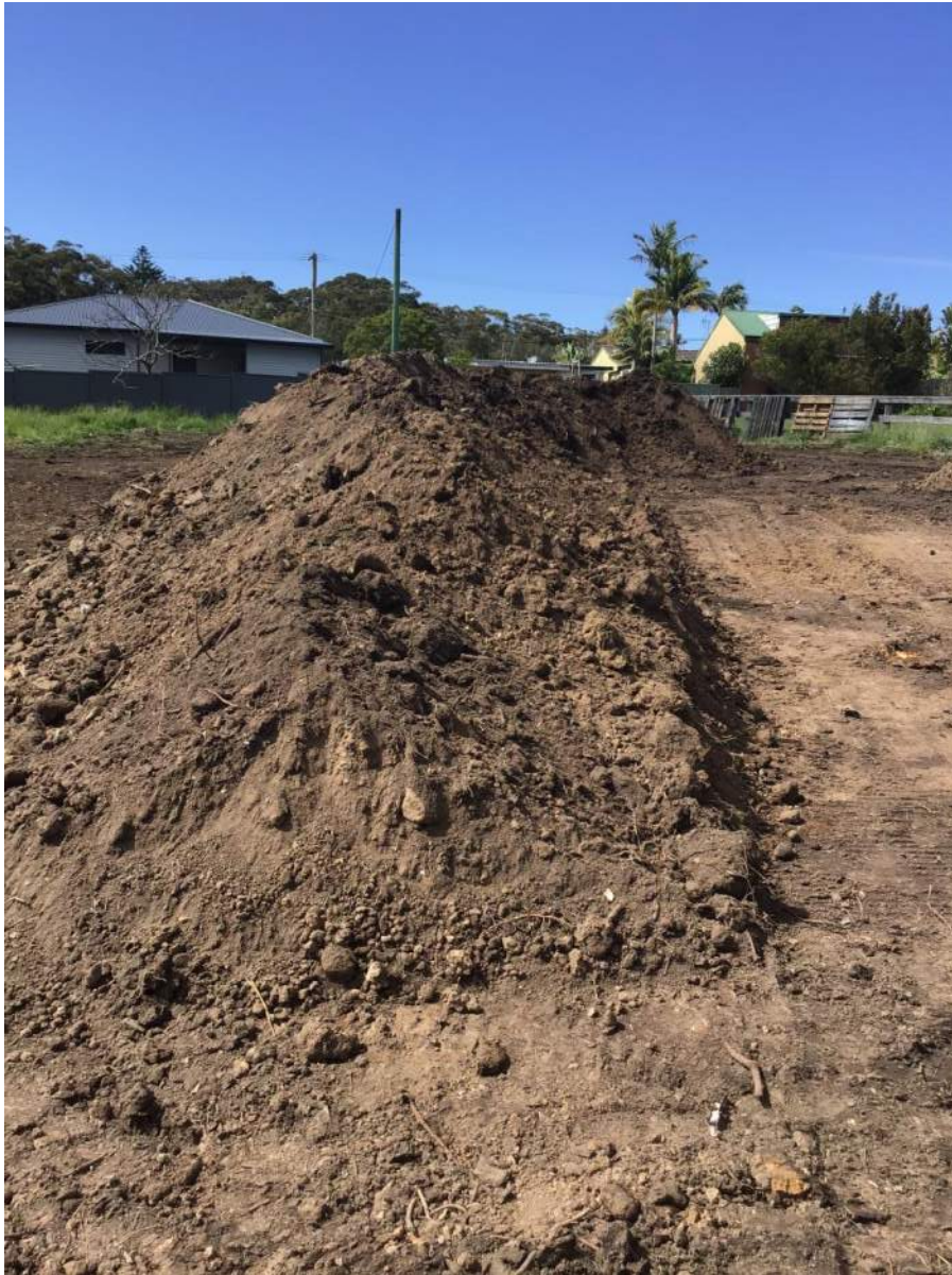
Photograph 7: Recent Stockpile Dumping (see OIN 10 on Figure 2 in Appendix A).
