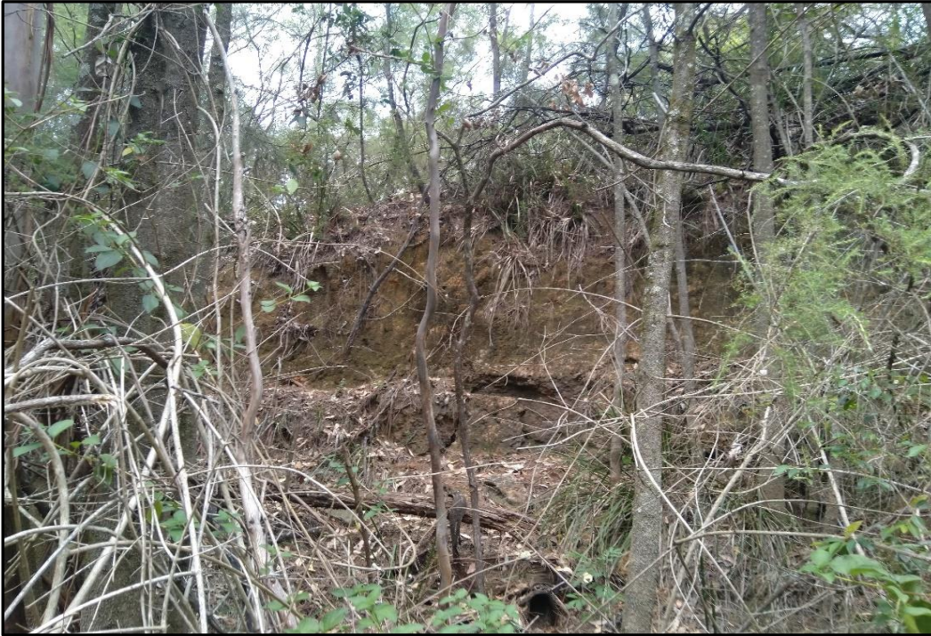
Photo 23: View of cutting showing loose soil wedges
