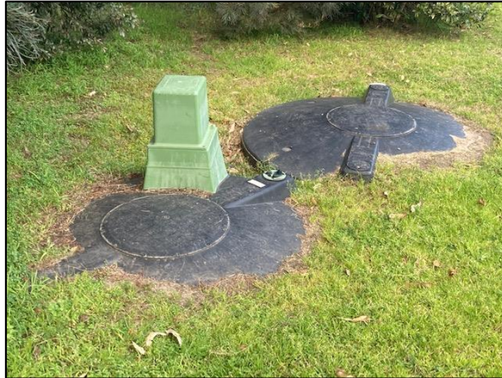
Plate 15 Wastewater Treatment Tank - Administration
