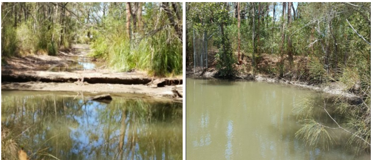
Photo 5: Concrete weir adjacent to the site and earthen weir opposite the site
