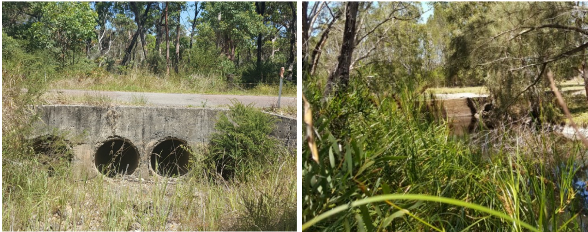
Photo 4: Chain Valley Bay Road culvert and concrete weir upstream of the site boundary
