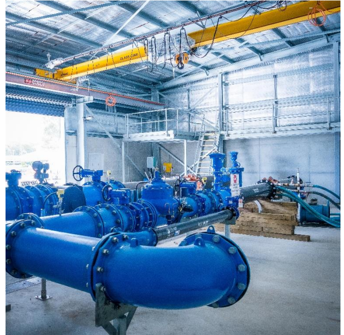
Image: Inside the Valve House on Albert Warner Drive during works (now completed)
