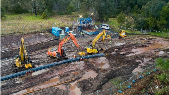
Image: Pipe in place to be pulled under Wyong River and Porters Creek
