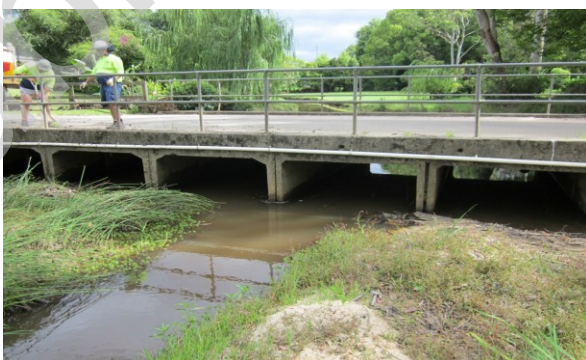
Photo 2: Debris under Tall Timbers estate access road
